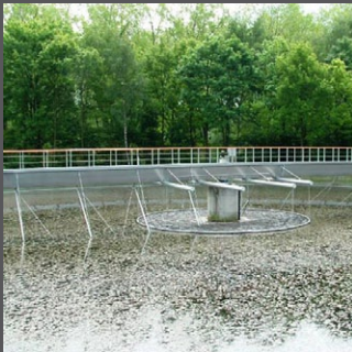
Slip ring assembly on a Circular Scraper Bridge
